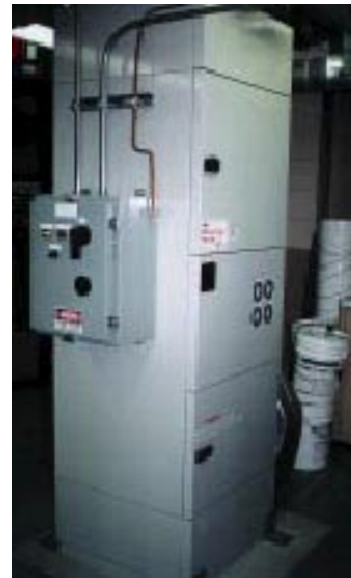
Circul-Aire APS-1000 complete with control system at B.C. Hydro Facility in Vancouver, B.C.
