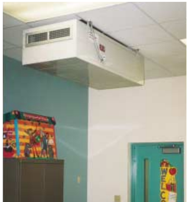
Typical Primary Learning Center classroom incorporating a ceiling suspended APS-400
