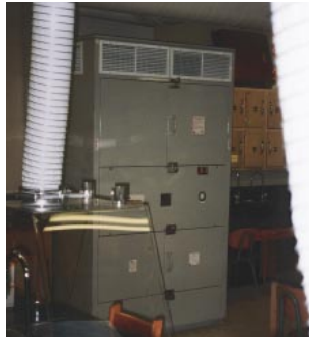
Source Capture Hood System attached to A.P.S.-3000
