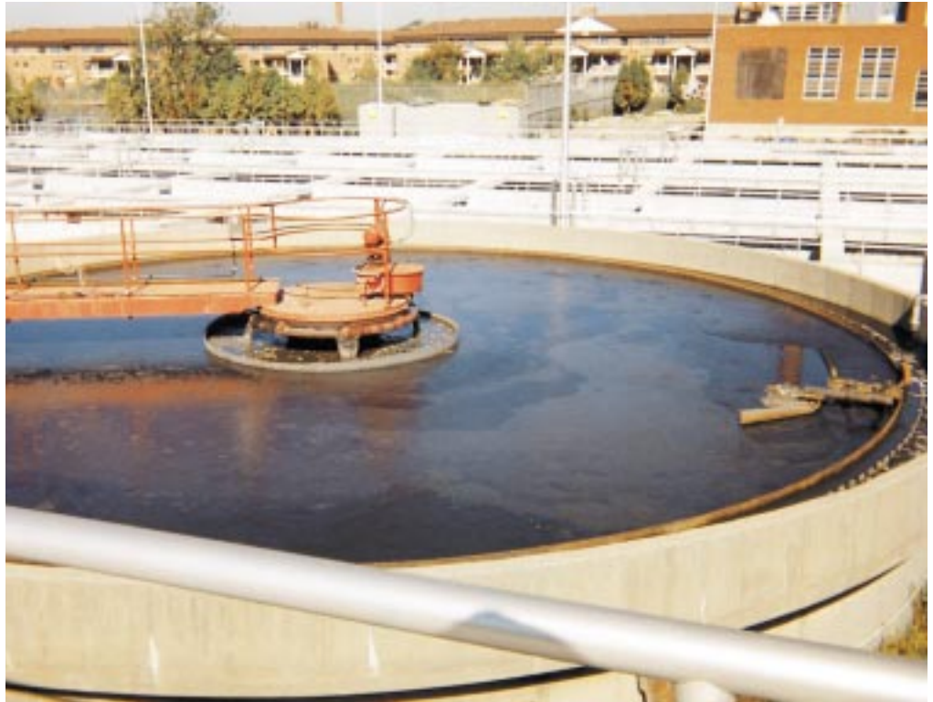
Waste Water Sludge Settling Tank
