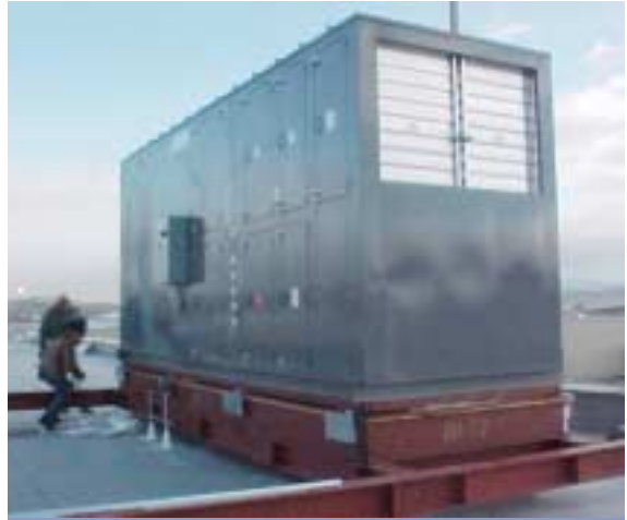
▲ Circul-Aire TMP-15000 unit on airport roof
