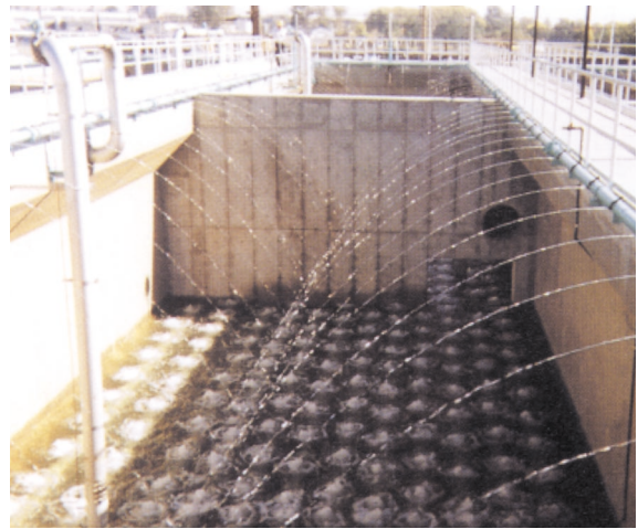
▲ Sewage Treatment Aeration Process
